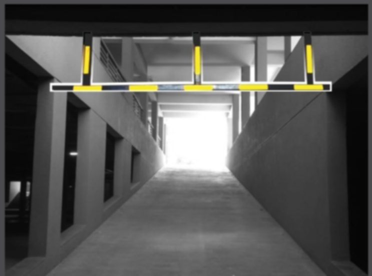
HEIGHT BAR FOR BASEMENT RAMP 2295
