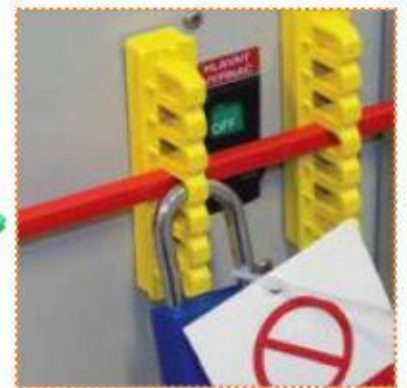
Group Circuit Breaker (LS-BR27)
